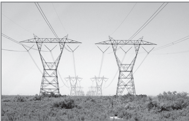
These tall towers hold up transmission lines. Transmission lines carry electricity from power plants to cities and towns.
